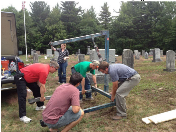
Daniel C. Patrick, Meghan Long, President Lee Atkin, Dick Hann, and Jeffrey Francom putting the foundation base of the headstone hoist
