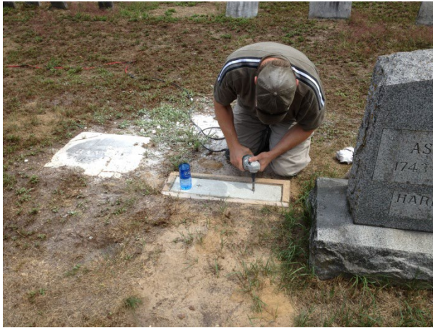
James Long preparing the four feet deep foundation for the headstone which will enable it up to endure the harsh winter conditions of northern New York.
